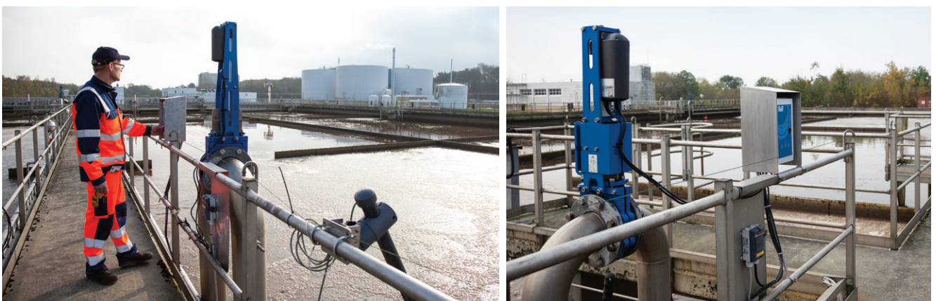
Aeration tanks at DIN Forsyning, Esbjerg.
