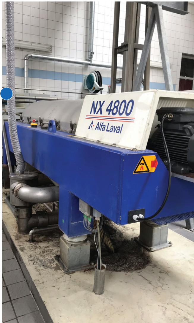
Decanter Centrifuge with LINAK actuators at Egaa wastewater treatment plant.
