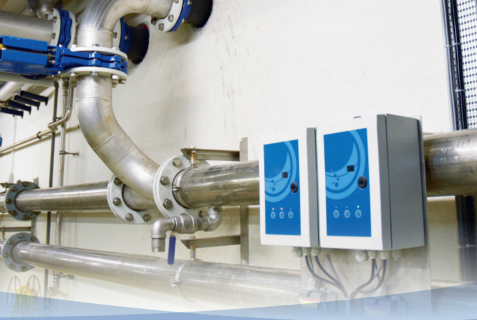
The transportation of fermented sludge to a buffer tank. Two WCUs are mounted on the wall where they are easy to access for the wastewater operator.
