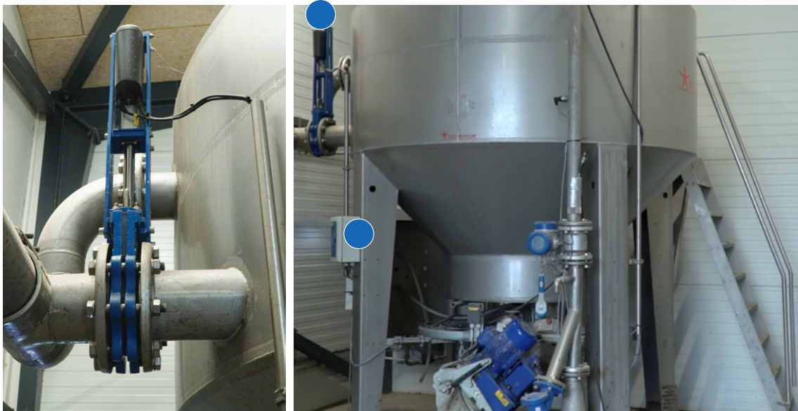
Stjernholm sand washer application. The control unit is mounted externally which makes it easy for the operator to access.
