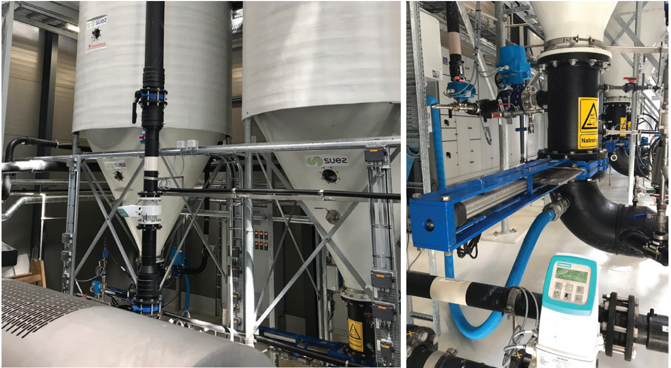
Three reactors with LINAK actuators at Marselisborg Wastewater Treatment plant.
