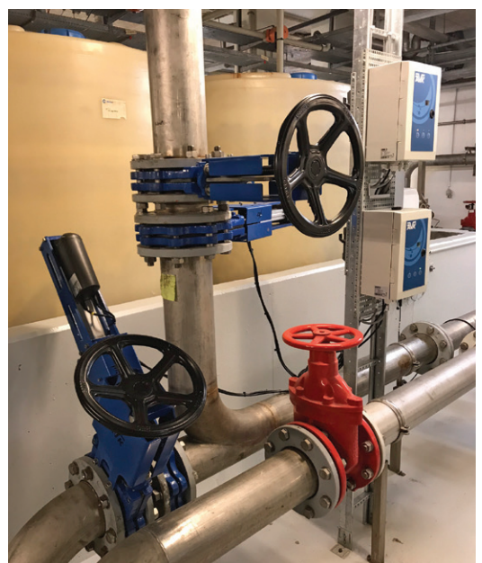
LINAK® actuators controlling the flow to the sludge buffer tank.
