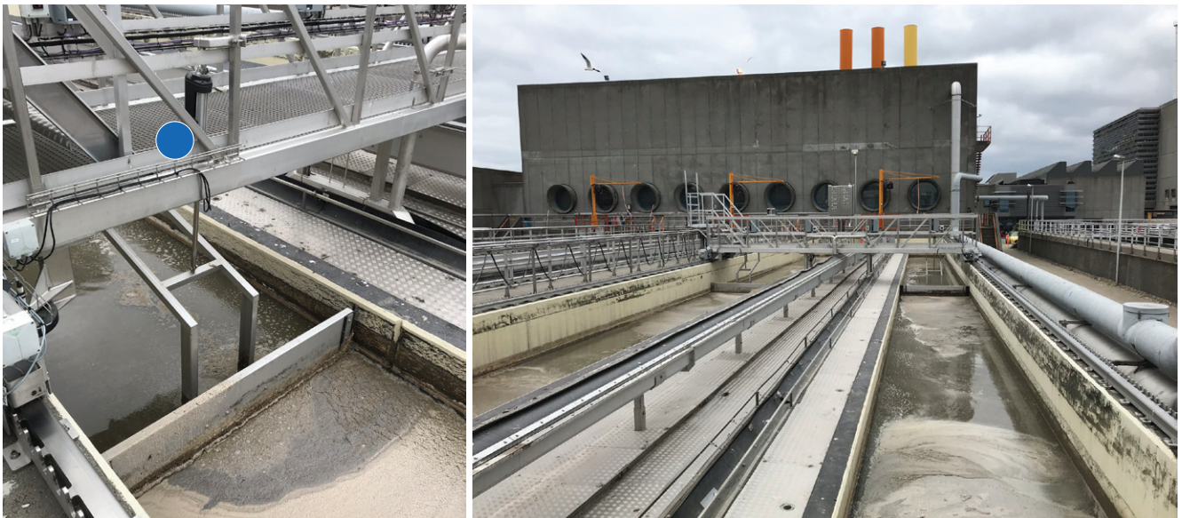
Biofos, Copenhagen, Grit Chambers – Oil and grease scrapers automated by LINAK actuator LA36.
